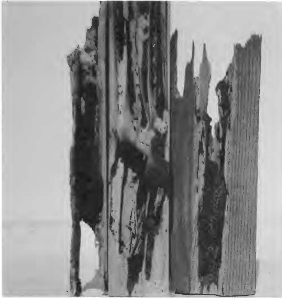
Figure 1. Portions of ceiling joists showing desert dampwood termite damage with fecal pellets glued together in the tunnels.
